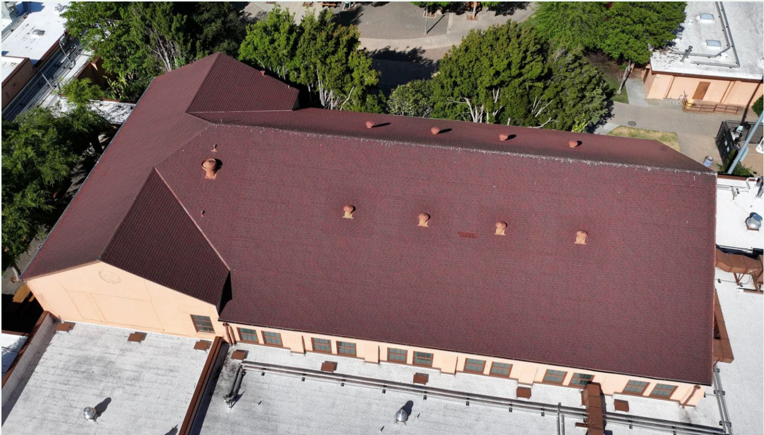
GYM 3 ROOF TO BE REPLACED
