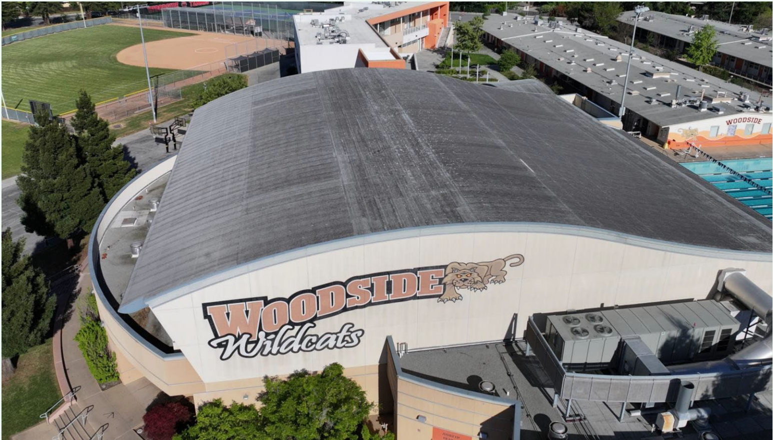
GYM ROOF TO BE REPLACED
