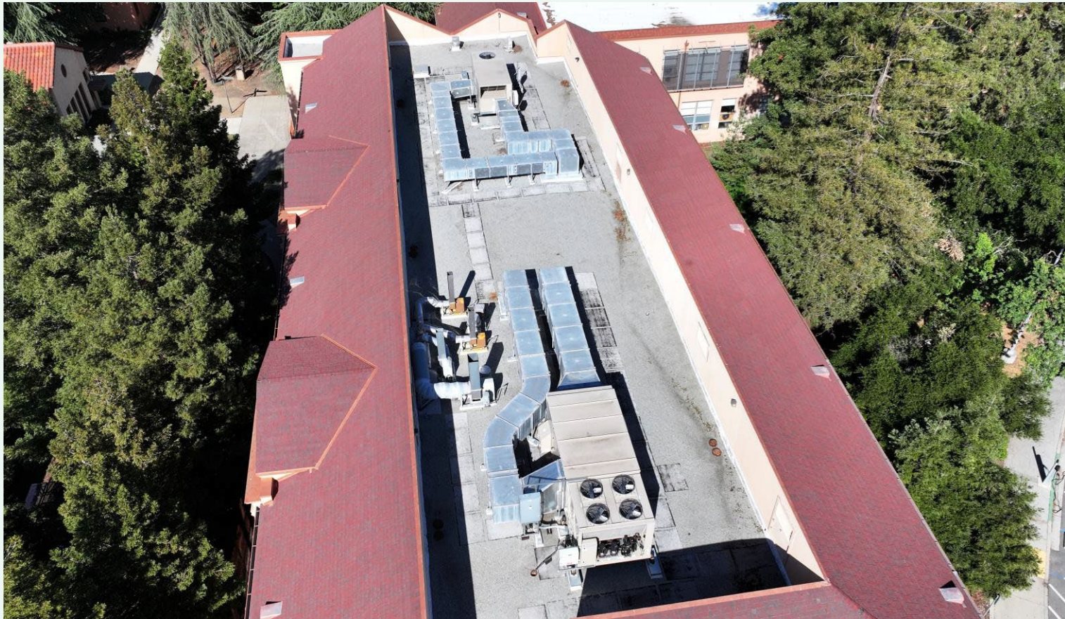
B-WING ROOF TO BE REPLACED
