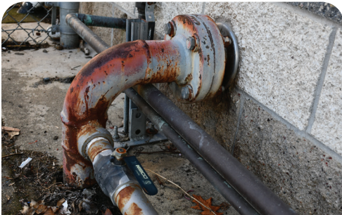
Rusty pipes need replacing
