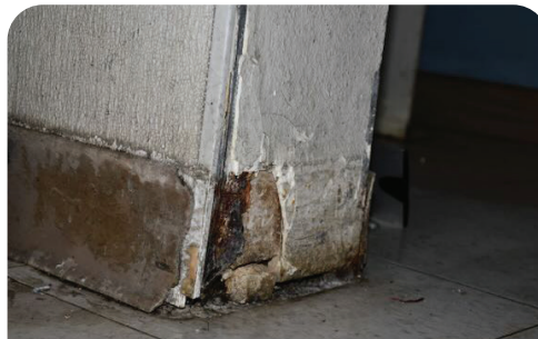
Deteriorating bathroom wall
