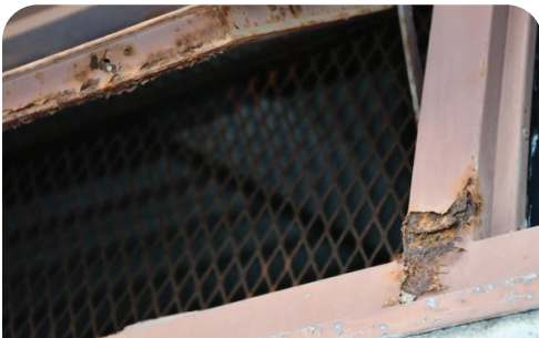
Decaying window frame
