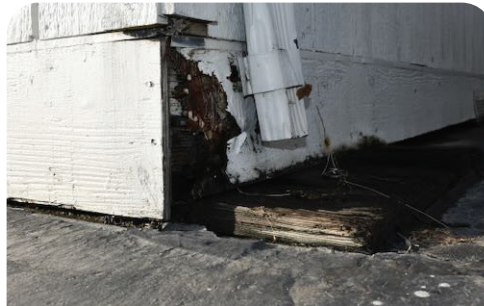
Classroom building dry rot
