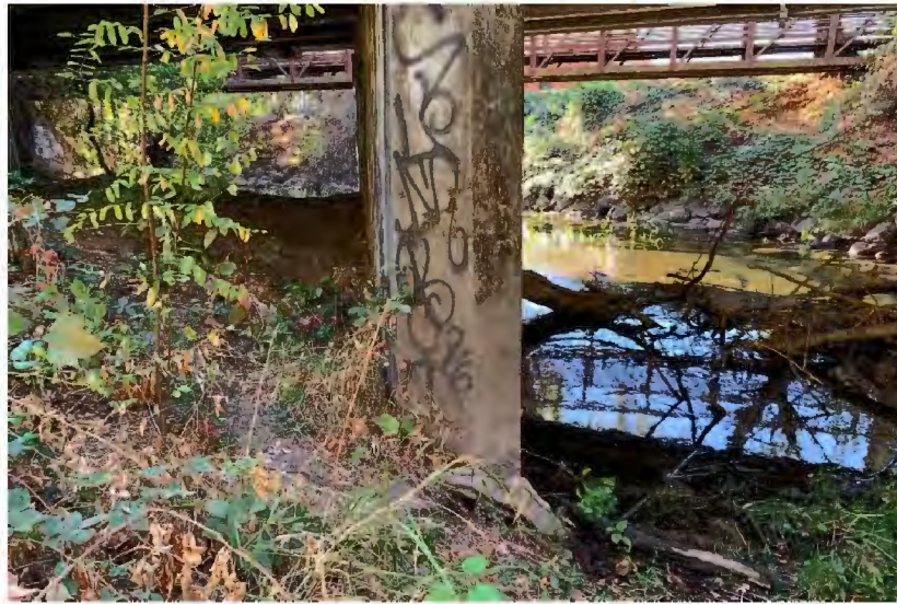
Figure 15: Site 9 Warner St Bridge Sediment Buildup (Looking downstream)
