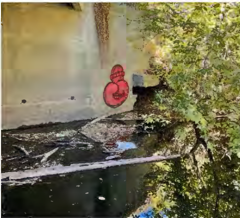
Figure 13: Warner St Bridge Scour
