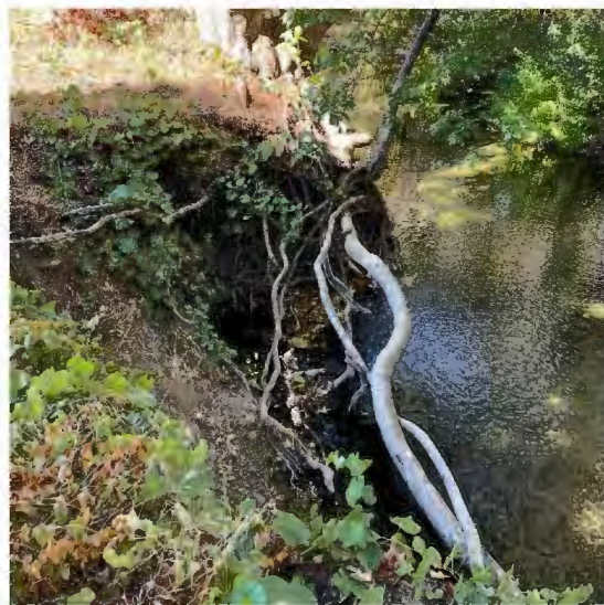
Figure 7: Site 4 Erosion and Characteristics (Looking downstream)
