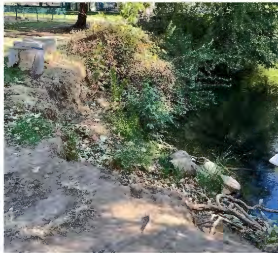
Figure 9: Site 6 Erosion and Characteristics (Looking upstream)
