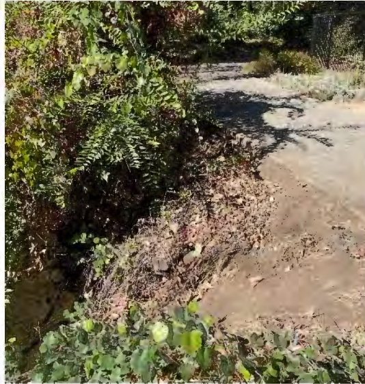
Figure 12: Site 9 Erosion and Characteristics (Looking downstream)
