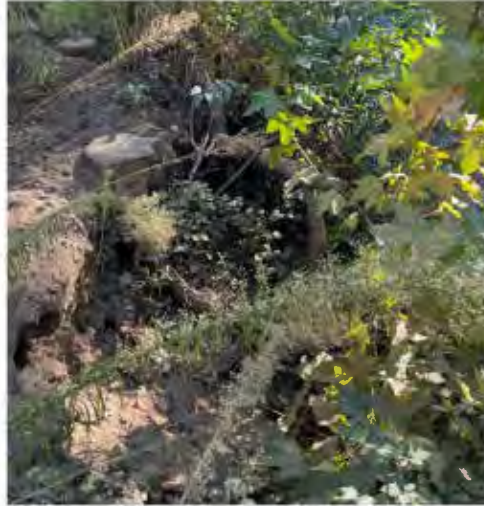
Figure 10: Site 7 Erosion and Characteristics (Looking upstream)
