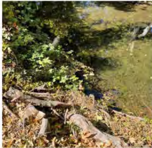
Figure 2: Site 1 Erosion and Characteristics (Looking downstream)
