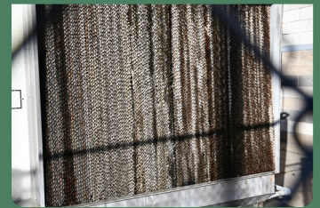
Outdated HVAC system
