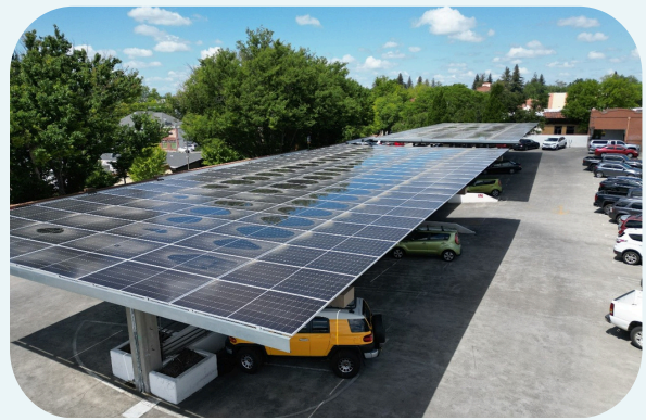
Solar Arrays at Parking Structure
