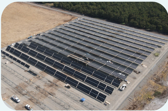
Solar Arrays at WPCP
