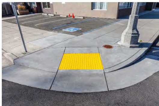
Source: Van Midde Concrete
