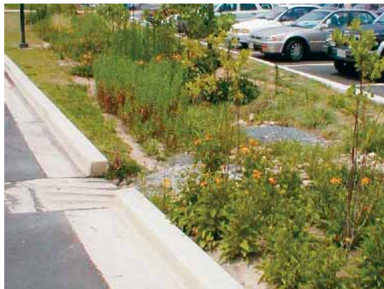
Grassy bio-swale with perforated curb.
