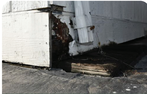
Classroom building dry rot
