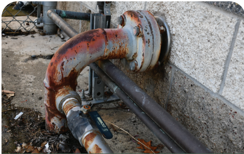
Rusty pipes need replacing
