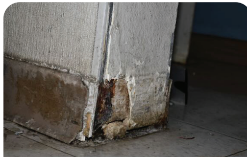
Deteriorating bathroom wall
