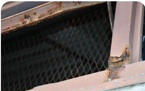
Decaying window frame
